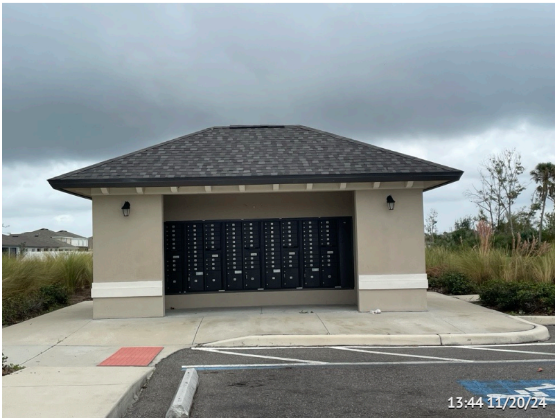
9th ST SE. Assigned To Clubhouse manager. The mailbox pavilion is well maintained.
